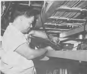
INSTALLING NEW multi-tubing in the Cat Cracker's control house is G. A. Berard, instrumentman A. He is hooking up individual pneumatic tubes to control instruments while the unit is in operation.
